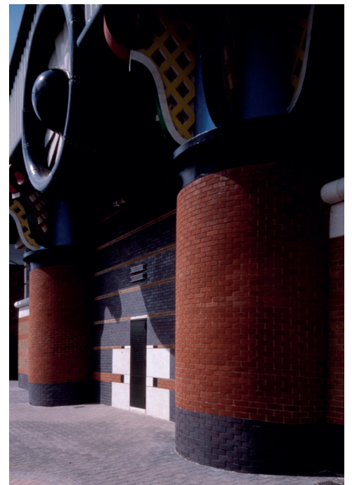
The IOD Pumping Station was part-buried into the embanked river's edge. The door has 'floated up' between its white jambs.
